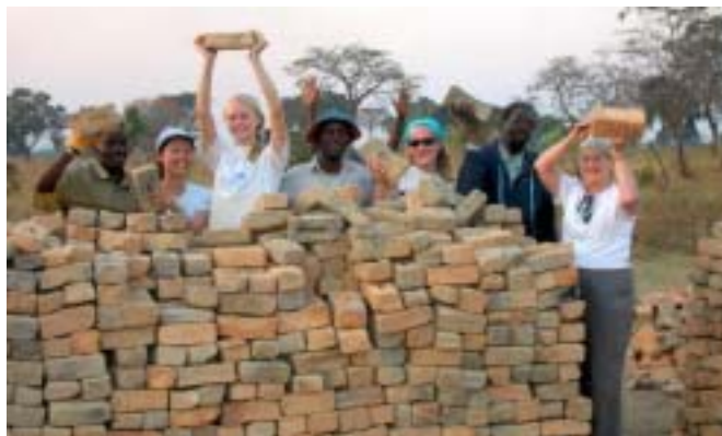
Above Faye Huang, Becky Rinearson Crowder, Cammie Samuelson, and Maria Haynes work with Zambian partners in Simukanka to sort some of the 40,000 bricks made by the villagers for the new medical clinic.
