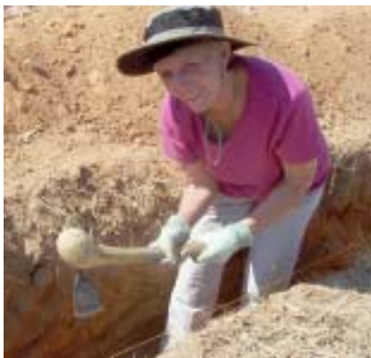
Here Nancy Friedman uses a traditional tool to help form the foundation for the new medical clinic in the rural village of Simukanka.
